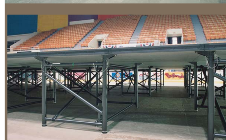
Large open spaces beneath the decks are ideal for stringing cables or stage-side storage.
